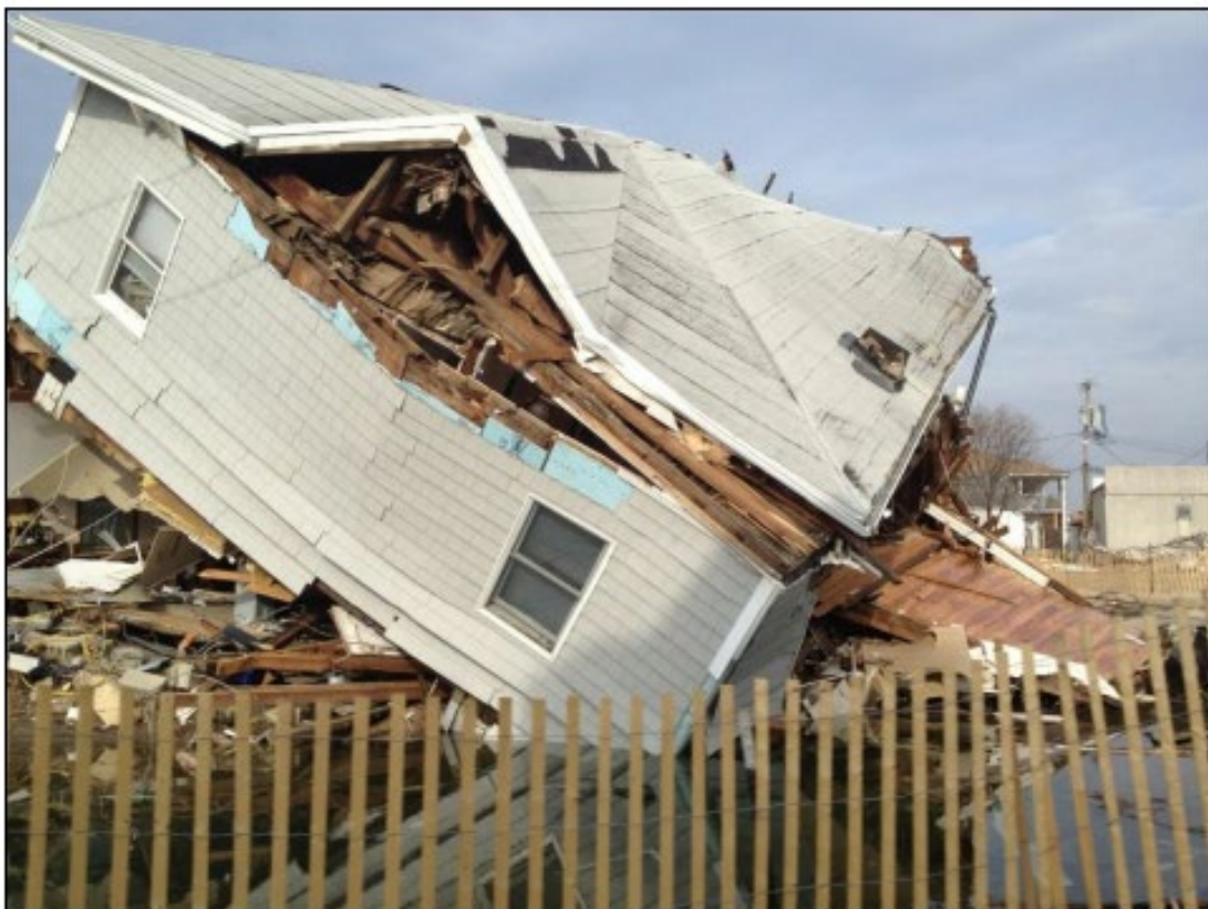
Image #4: The above example photo illustrates a building that is canted or wracked.
